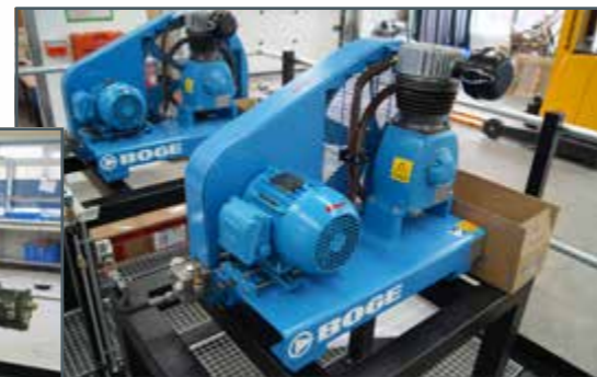
Compressed air station
