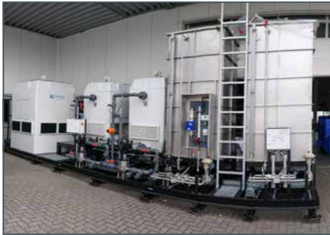
Outdoor wet cooling towers and receiving tanks for process water and ethylene glycol
