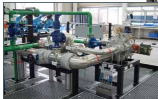
Steam driven auxiliary pumping station
