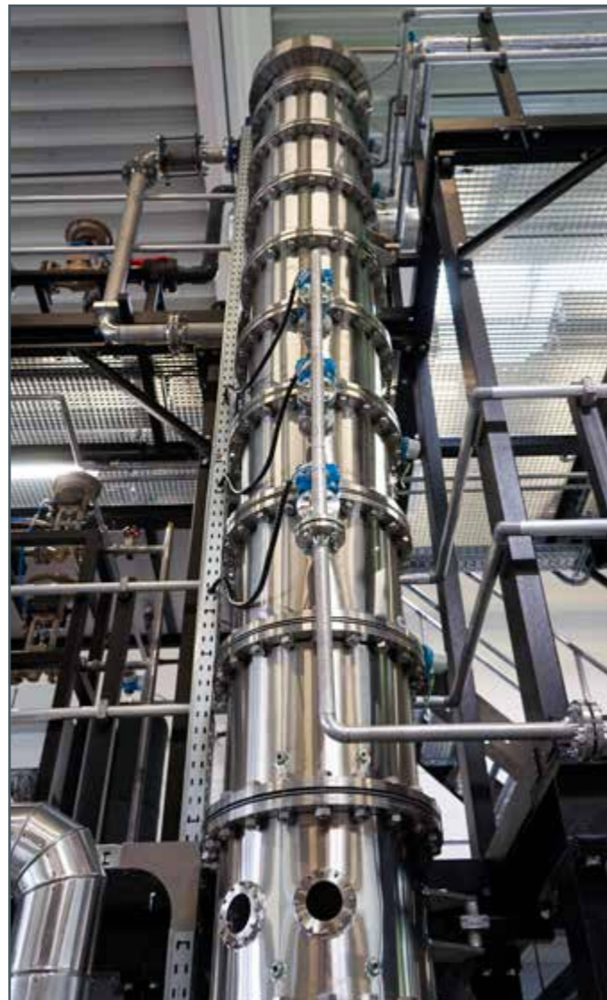
Distillation process: rectification column
