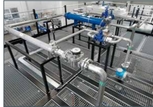
Thermal reactor with chemical injection system
