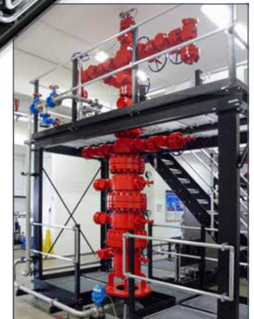
Wellhead and Xmas-tree
