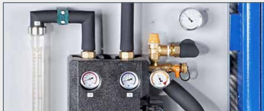
The solar circuit station contains a circulating pump and key components for safe operation.
