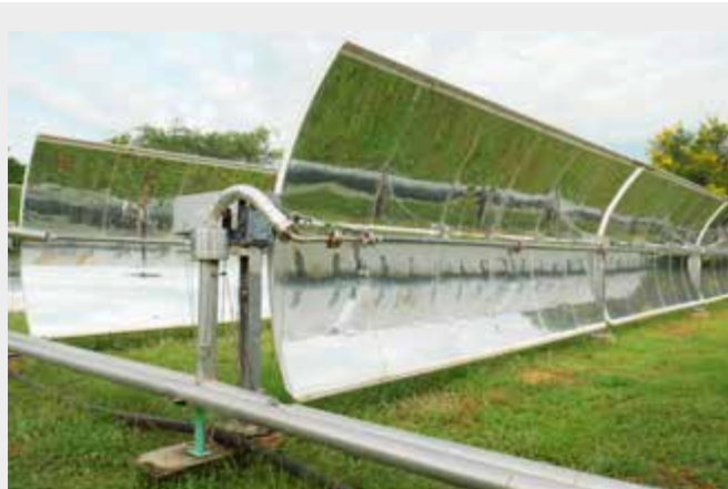
For a power plant, individual parabolic trough collectors can be connected in a collector field.
