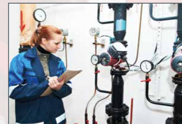
Checking the system components
