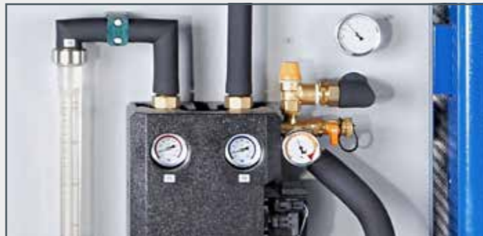
The solar circuit station contains a circulating pump and key components for safe operation.
