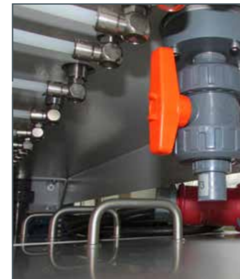
Pressure measuring points and drain valve
