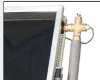
The controller regulates the circulating pumps and can be used to log data.
