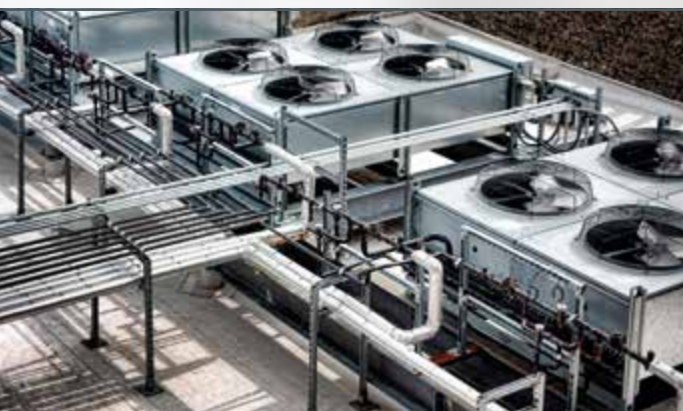
Condenser in a refrigerant network
