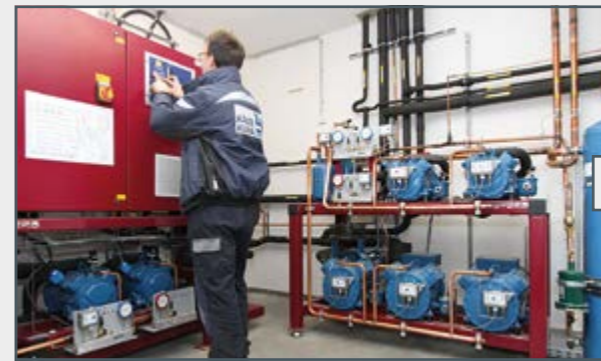
Installation frigorifique industrielle
